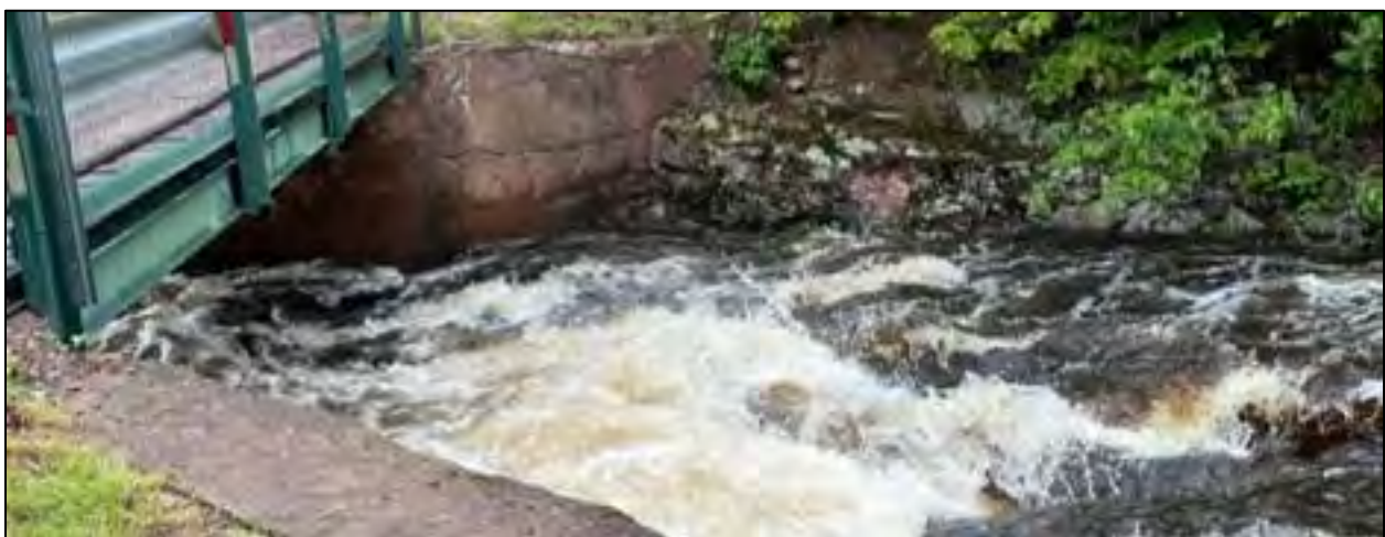
End of Reach 3 – Kimball Town Park bridge over Kimball Falls at 600 cfs
