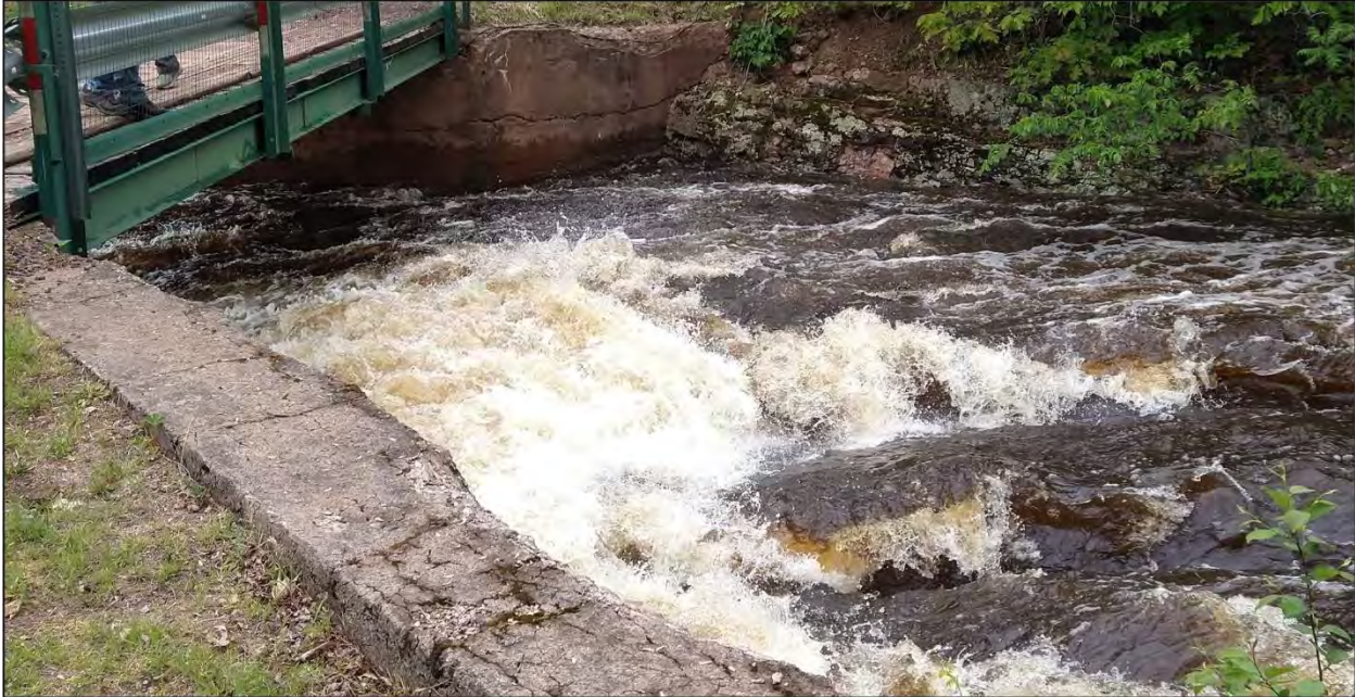
End of Reach 3 – Kimball Town Park bridge upstream of Kimball Falls at 1,200 cfs
